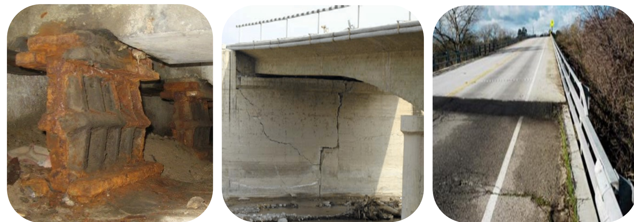
Figure 1. Common bridge problems: joint corrosion, cracking and approach settlement.
