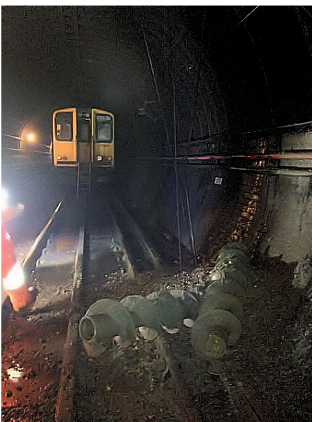
Figure 1: CFA auger sections found on the track after penetrating tunnel.
