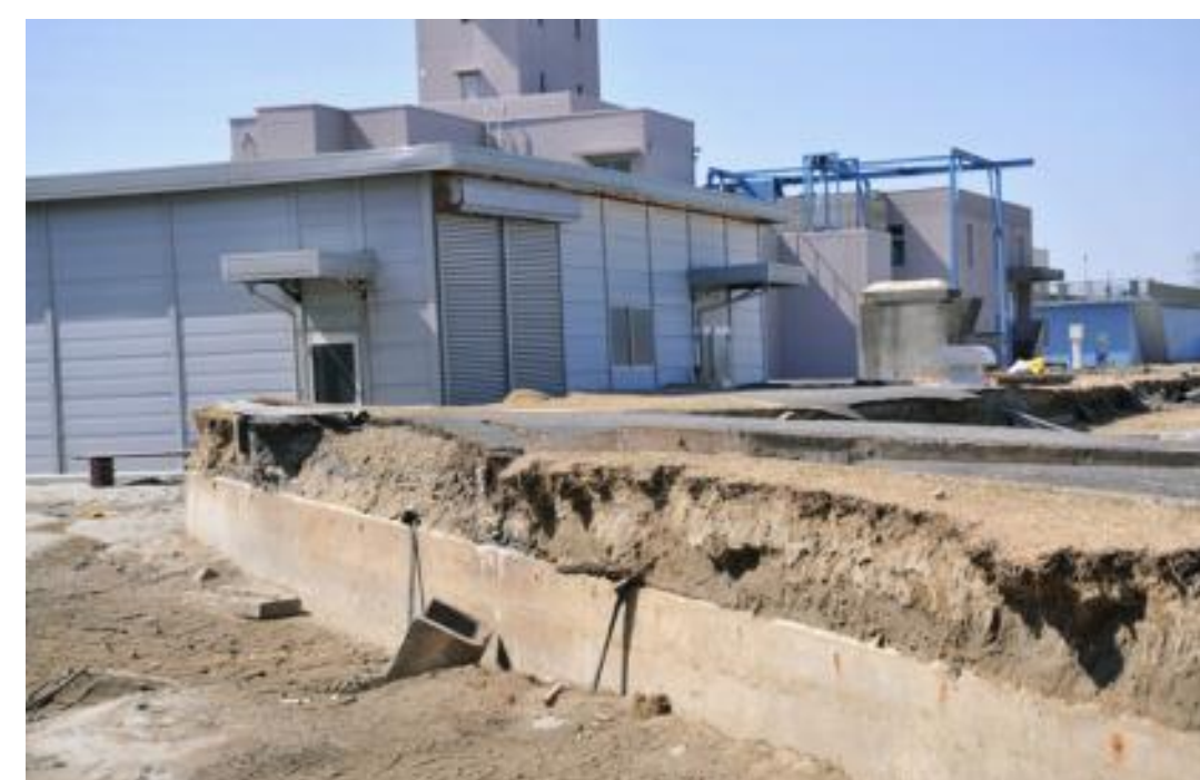
Figure 1. Uplift of buried conduit during 2011 Tohoku earthquake [2]
